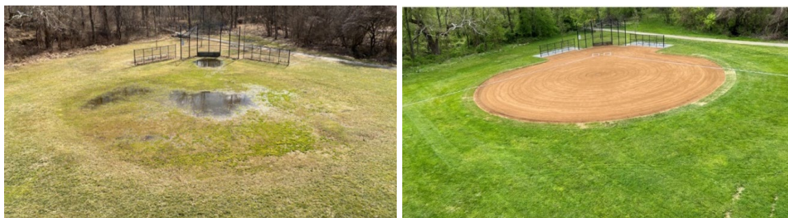
Before (left) and after (right) full mechanical renovation at Randolph Hills Local Park.
